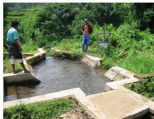
The majority of the civil structure was still in good condition and could be put back into operation for the MHP relatively easily.
